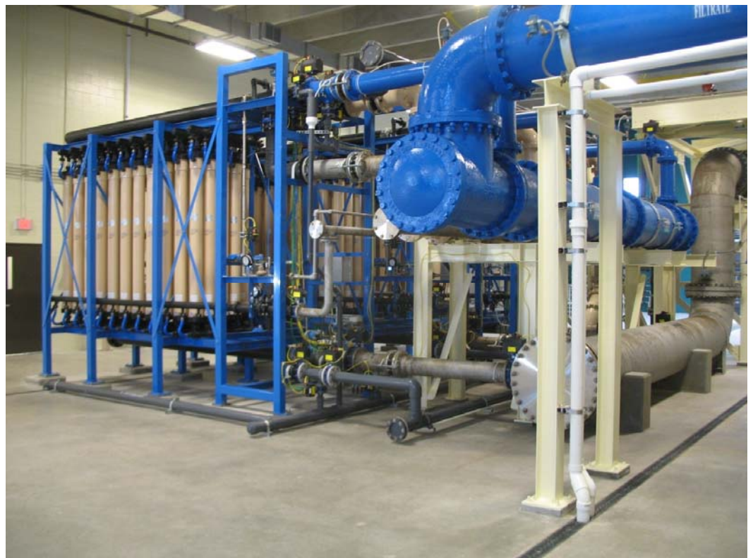
Photo: Plum Creek Water Purification Facility in Castle Rock
